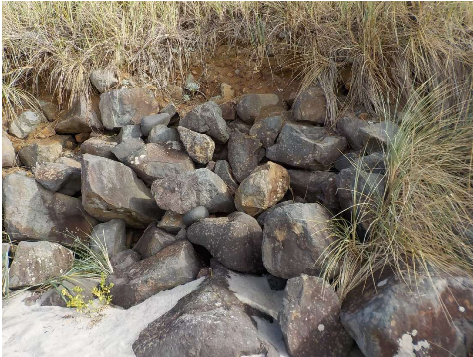
Photo 6 – View of the damaged riprap revetment exposed at the base of the bluff slope.
