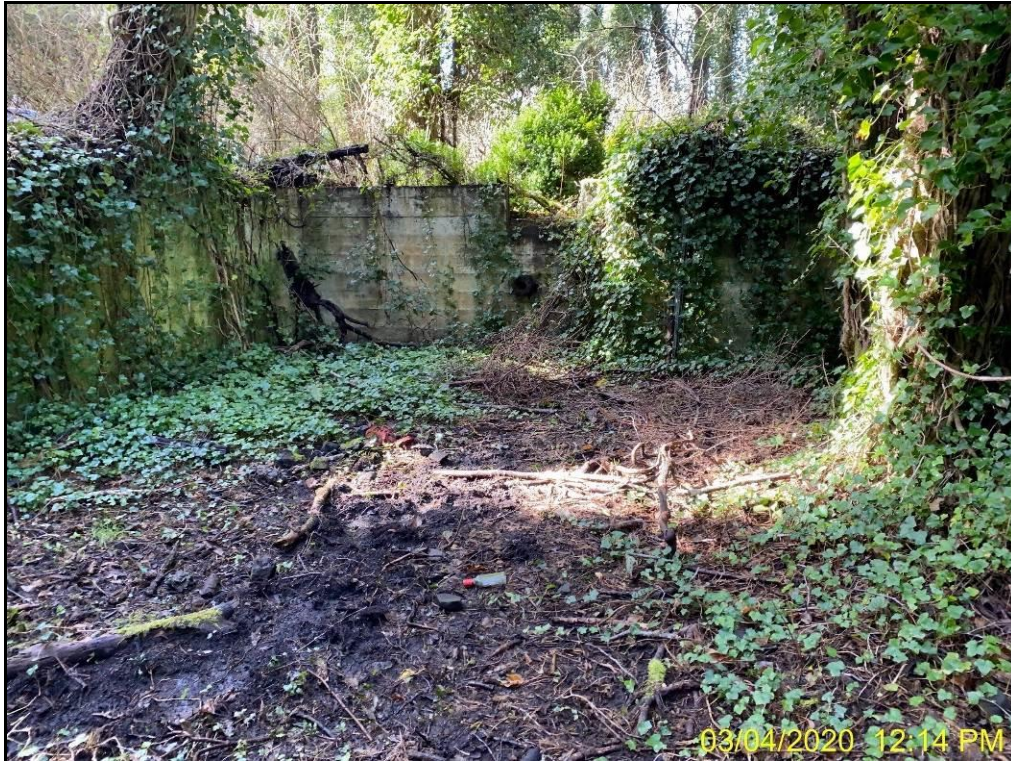
Photo 6: Retaining wall with a large drain pipe near where old residence had been.
