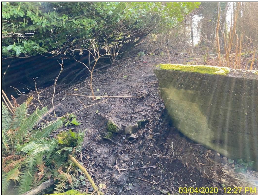
Photo 7: Looking southeast at failed retaining wall near where driveway had entered property from the west.
