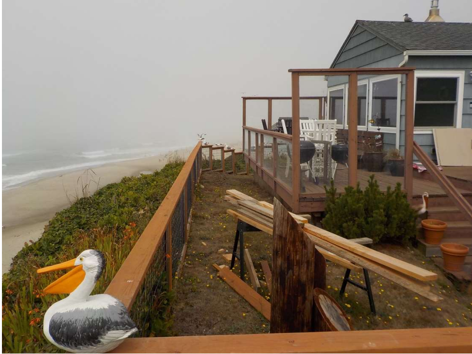
Photo 3 – Northerly view of the western side of the existing house, deck and bluff edge
