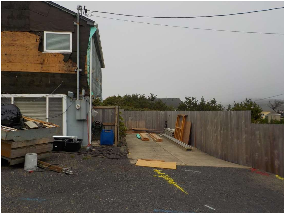
Photo 2 – Northerly view of the area proposed for construction of the attached carport addition.
