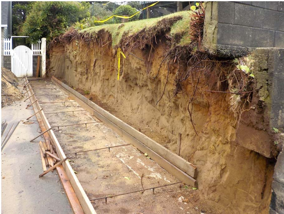
Photo 2 – View of the cut slope and area proposed for the retaining wall.
