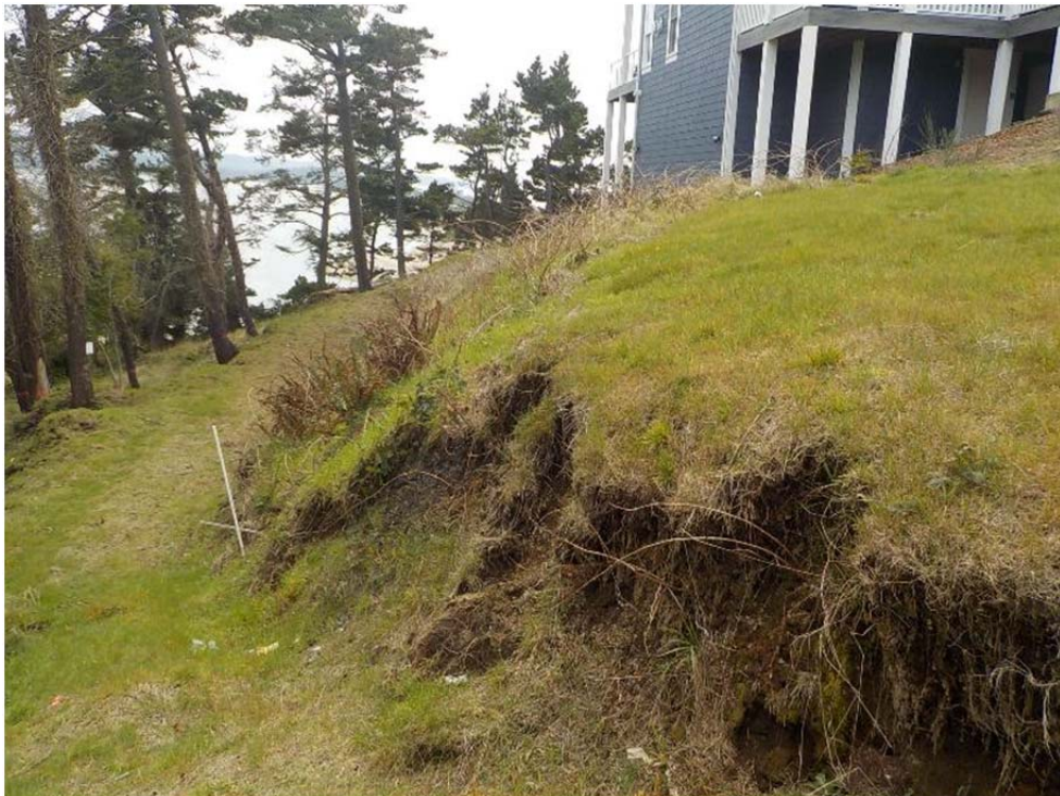
Photo 4 – Southerly view of Tax Lot 1800. Note the unretained cut slope.
