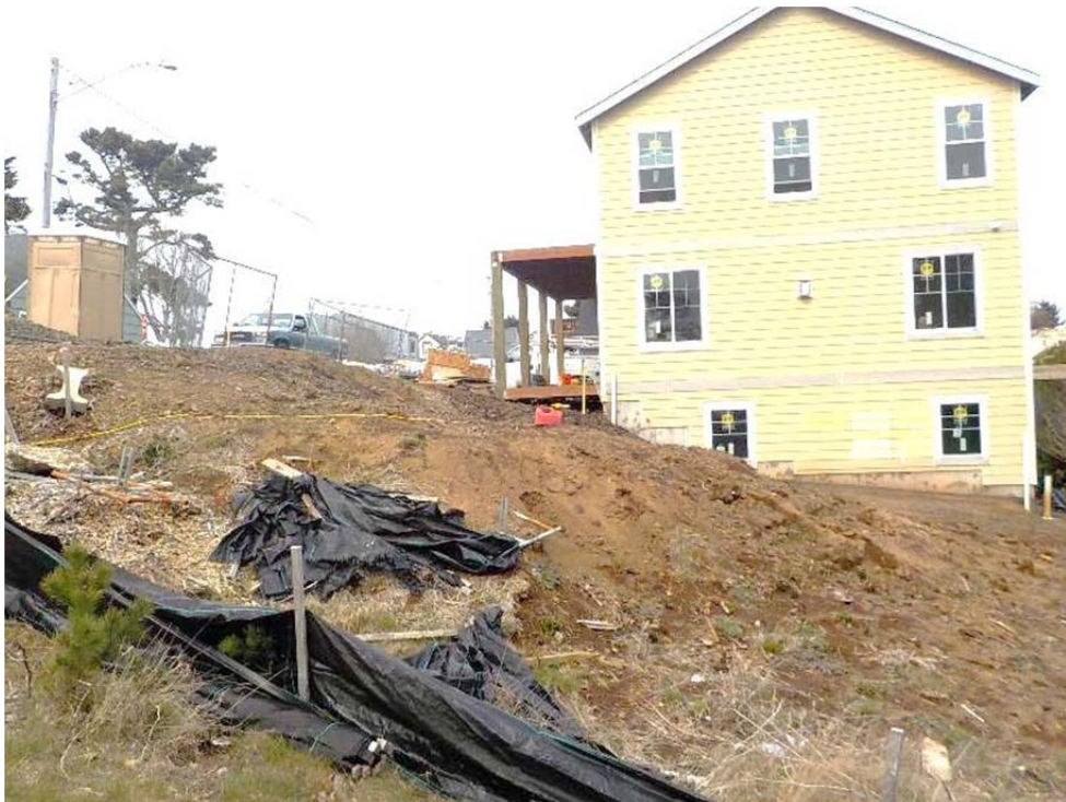
Photo 2 – Northerly view of Tax Lot 1300. Note the stockpile of fill soil and debris.
