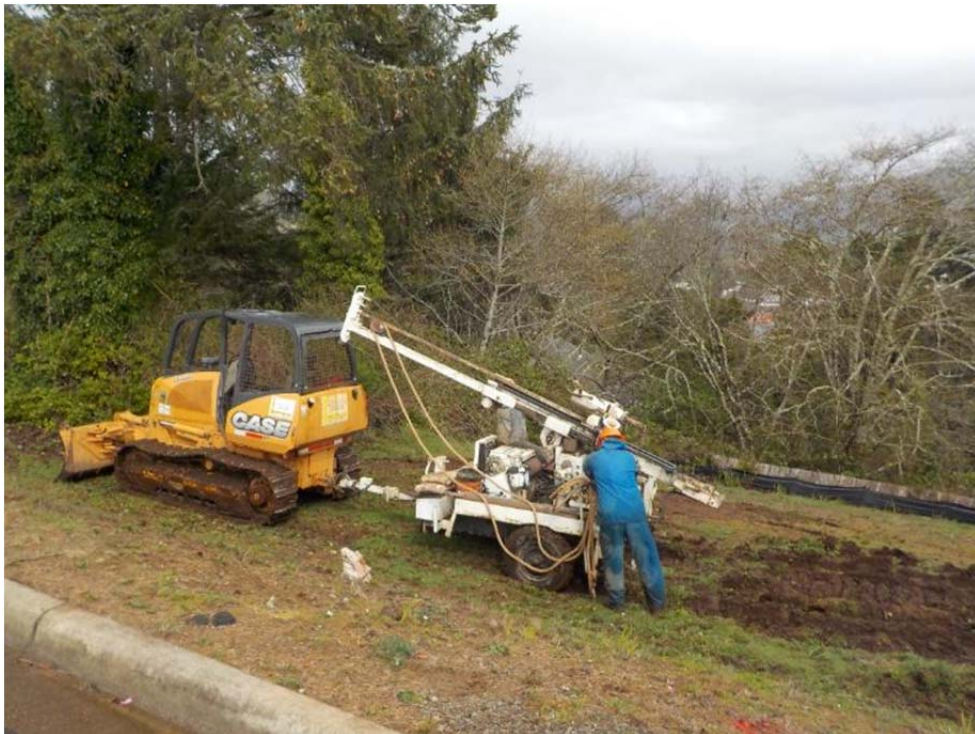
Photo 16 – View of the drill rig set up on Tax Lot 1300 during subsurface exploration (4/12/2018).
