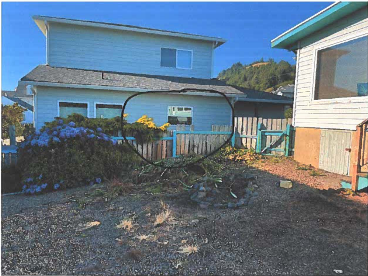
Photo of fence in backyard – notice where the top of the boards have broken off.
