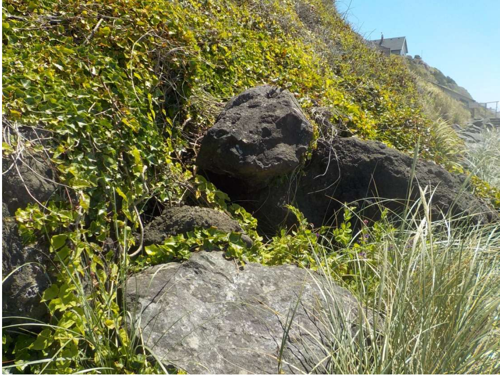
Photo 3 – Close-up view of the existing rip rap stone along the base of the bluff.
