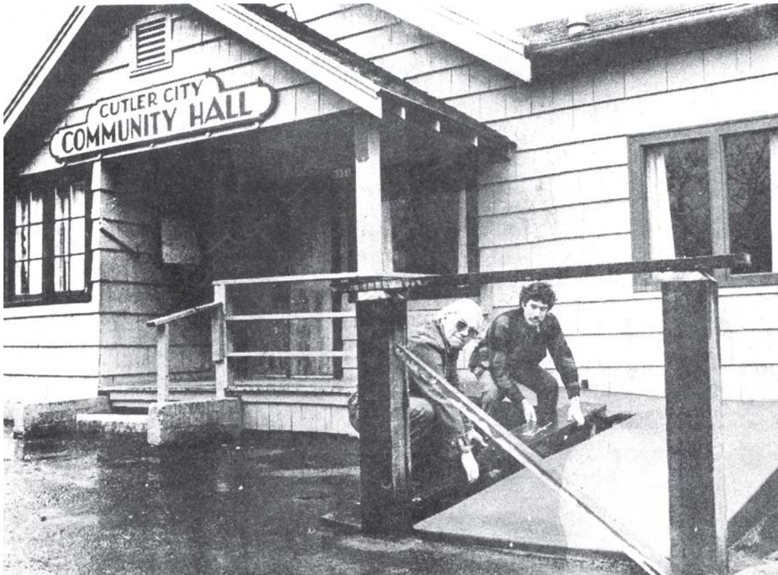
Ed Johann and Bob Barden construct access ramp for Cutler City Community Club
